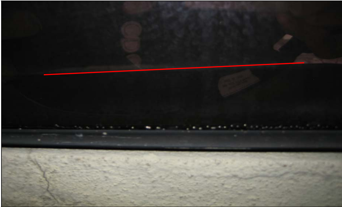
Photo #007: Exterior view looking through the glass at the talcum powder. A clean, straight line indicates no visible adhesion failure between the VHB-SGT and glass.
