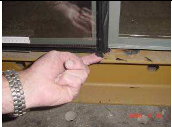
Photograph 4.6: Details of the silicon condition for the last displacements cycles in sample 1
