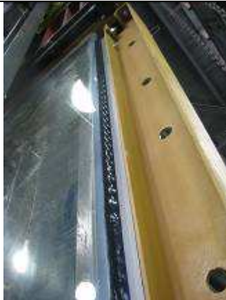
Photograph 4.5: Details that shows deformation of the silicon located in the vertical joints between modules and in their connections with the sides profiles.
