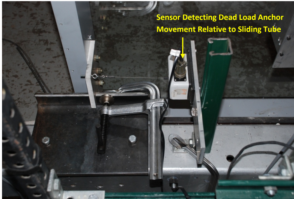
Figure 17- Sensor on Dead Load Anchor
