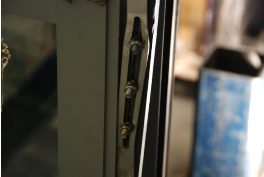
Figure 33- Widening of Slotted-Holes
