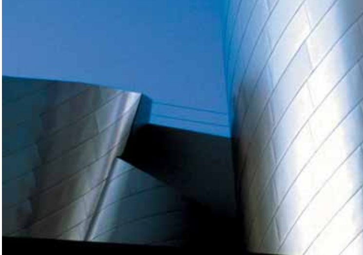
Walt Disney Concert Hall, Los Angeles, CA, USA Architect: Frank O. Gehry Curtain wall: Permasteelisa, 2003 Stiffener and frame attachment.
