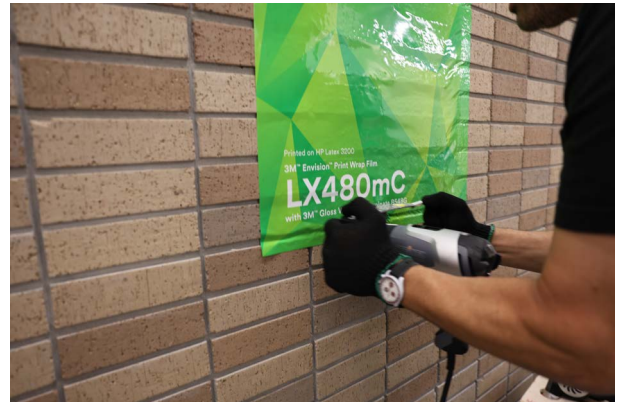
Figure 8. Lean into the wall to achieve consistent pressure on the TSA-4 tool.
