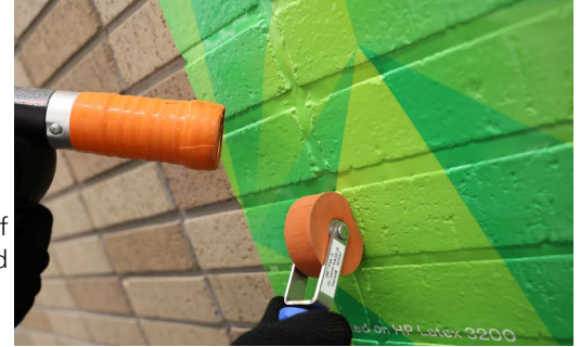
Figure 15. Use the TSA-3 tool and heat gun to touch up poorly adhered areas.
