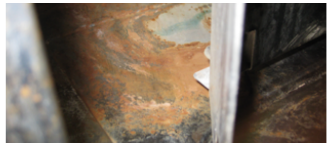
A combi-oven showing corrosion.
