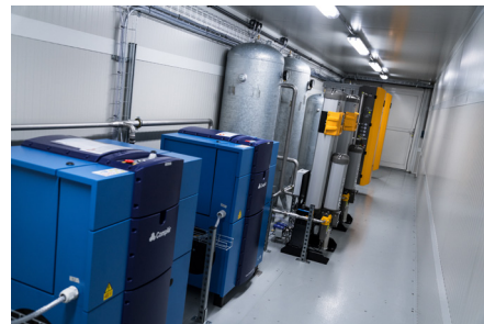
Picture 2: Nitrogen generation system in Power plant container system Courtesy of Jotem Waterbehandeling BV, NL
