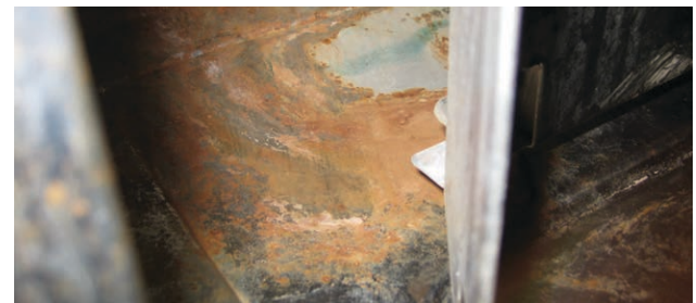
A combi-oven showing corrosion.
