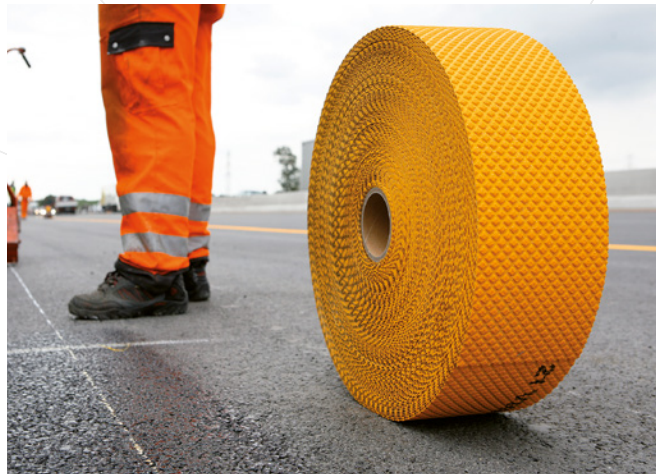
Removable, temporary pavement markings
