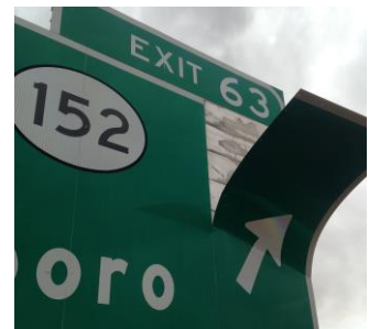
flat panel aluminum construction – panel that has broken away
