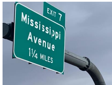
flat panel aluminum construction – lettering fail at panel seam
