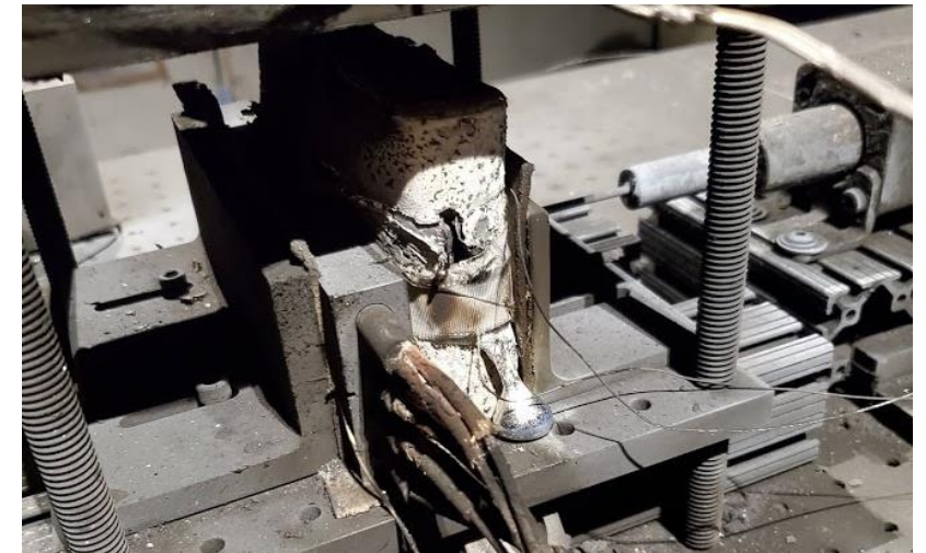
Thermal initiated runaway resulting in melted containers
