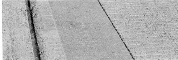
Figure 8. Portland cement concrete groove with a light corduroy pattern, made with properly spaced gang-stacked diamond cutting blades.
