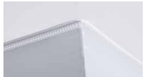
3M™ Clear Track Hallway Fiber Pathway installed around exterior corner
