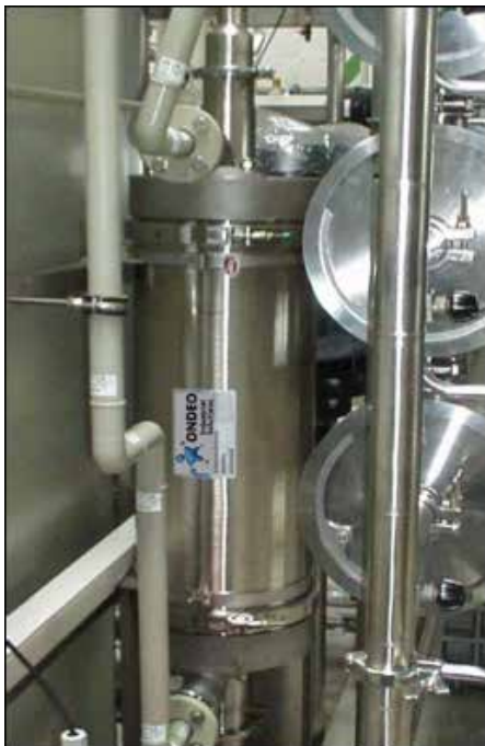
Contactors in an 8 m 3 /h ROCEDIS plant
