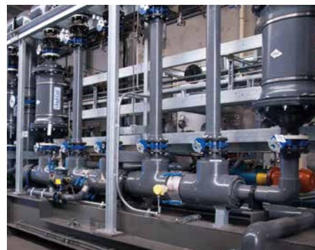
Figure 3. 3M™ Liqui-Cel™ EXF-14x40 Series Membrane Contactor in CSG Pilot Degassing System
