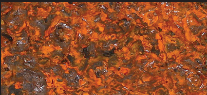
Without corrosion protection treatment
