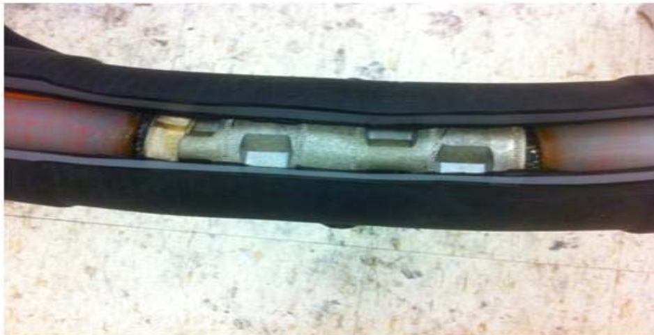
Figure 3. Sample B Inspection of Connector and Cable Insulation After Load Cycling
