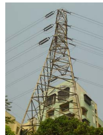
TATA Power Borivali to Malad 110 kV Line
