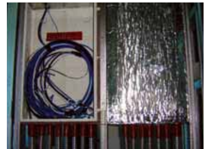
Low voltage electrical boxes for a very large construction project in Las Vegas were firestopped on five sides with 3M™ Interam™ Endothermic Mat. Segments were attached with adhesive, and seams sealed with aluminum foil tape.
