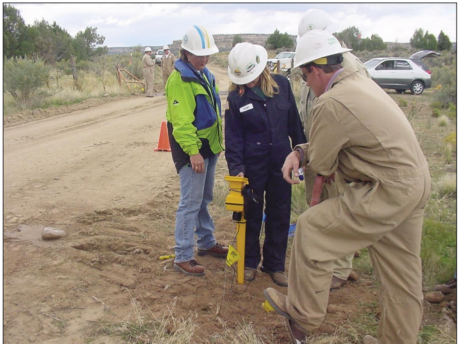
Marker read-write units load the ball location relative to the pipe, ID number, GPS coordinates, and any other identifying information onto the ball before burial. The same units will later use this information to confirm the precise location and depth of each marked crossing (Fig. 5).
