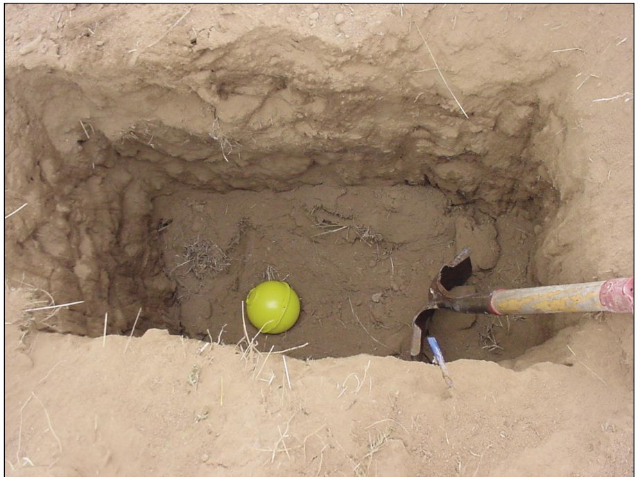
Backfilling the exposed pipes to a measured level allows placement of the ball marker at a known distance from the pipe (Fig. 4).
