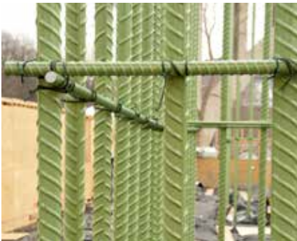
Rebar coated with 3M™ Scotchkote™ FBE Coating 413 being used in a bridge project
