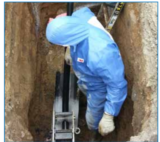
Retrieving the spray head in Veolia, Prague's third 3M™ Scotchkote™ Pipe Renewal Liner 2400 project.
